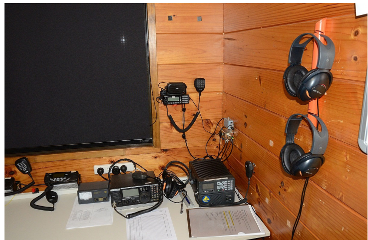
The HF Radio installation at 400 East Coast Road
