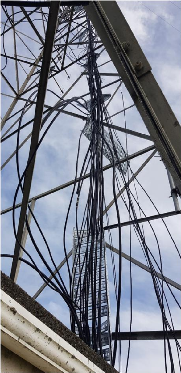
Cables broken away from the trays.
